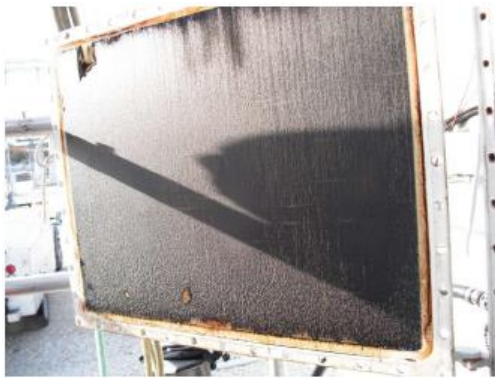
Sludge On Inside of Door
